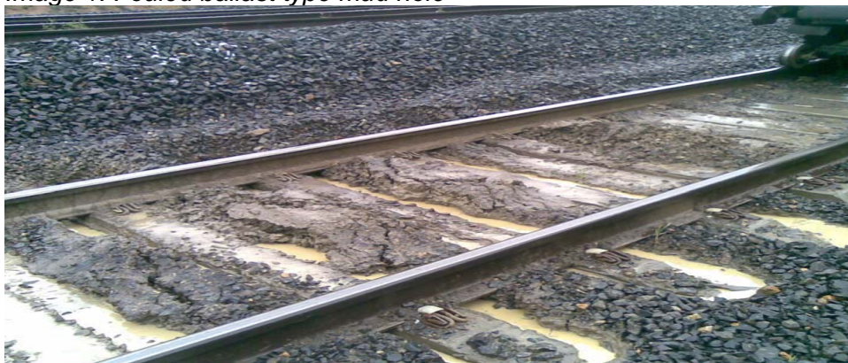
Image 1: Fouled ballast type mud hole
