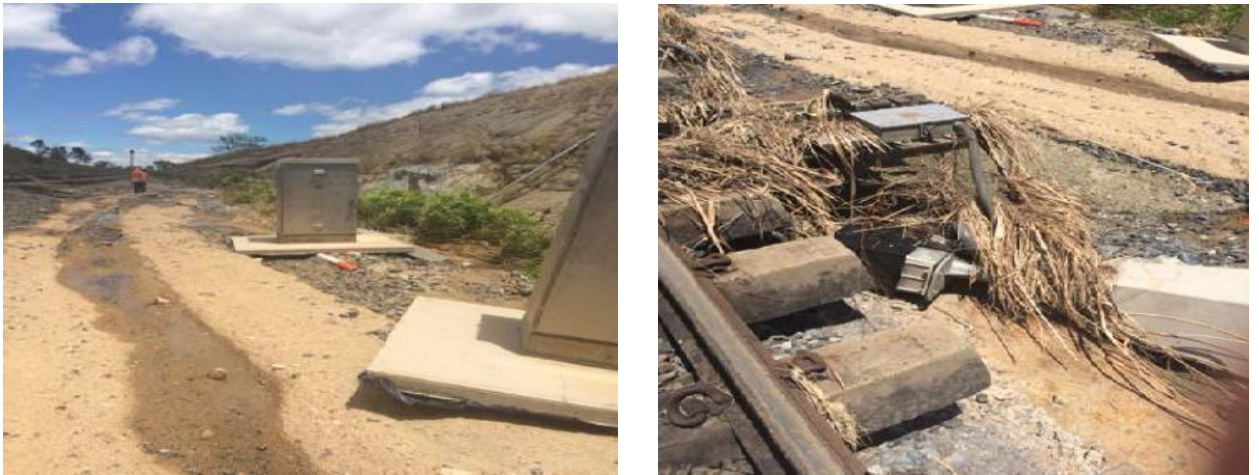
Figure 10 Points, Signals and Electrical Boxes at Fry (89.740km)
