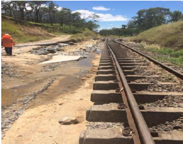
Figure 7 Track and Formation Damage at Fry (89.550km)
