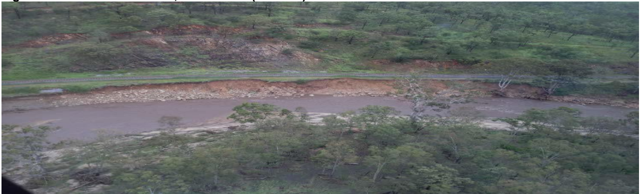
Figure 11 Scour at Bells Creek, Mt Rainbow (100.3km)
