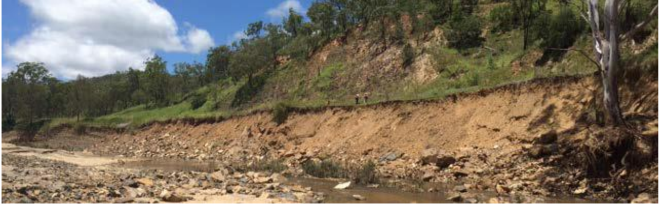
Figure 1 Scour at Bells Creek, Mt Rainbow (100.3km)
